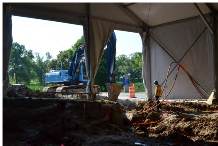
Figure 4.40. Temporary removal of a fiber-optic cable, June 25, 2013 (UWM photo on file, UWM-ARL).
