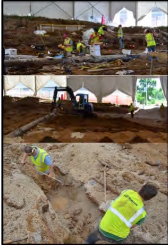
Figure 4.43. Working around the water main (top); removal of the water main (middle); checking for any remaining human remains or coffin wood (bottom) (UWM photo on file, UWM-ARL).
