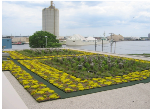
Figure ES-5. Green roof at the GLWI, which is used as a demonstration project to highlight strategies for mitigating stormwater runoff.
