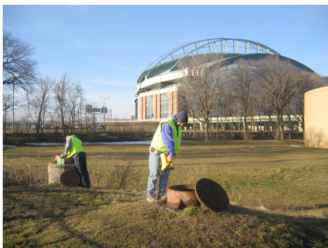
Figure ES-3. Dye testing of sanitary sewer lines near Miller Park. Testing for the human Bacteroides genetic marker was positive in a nearby stormwater outfall.
