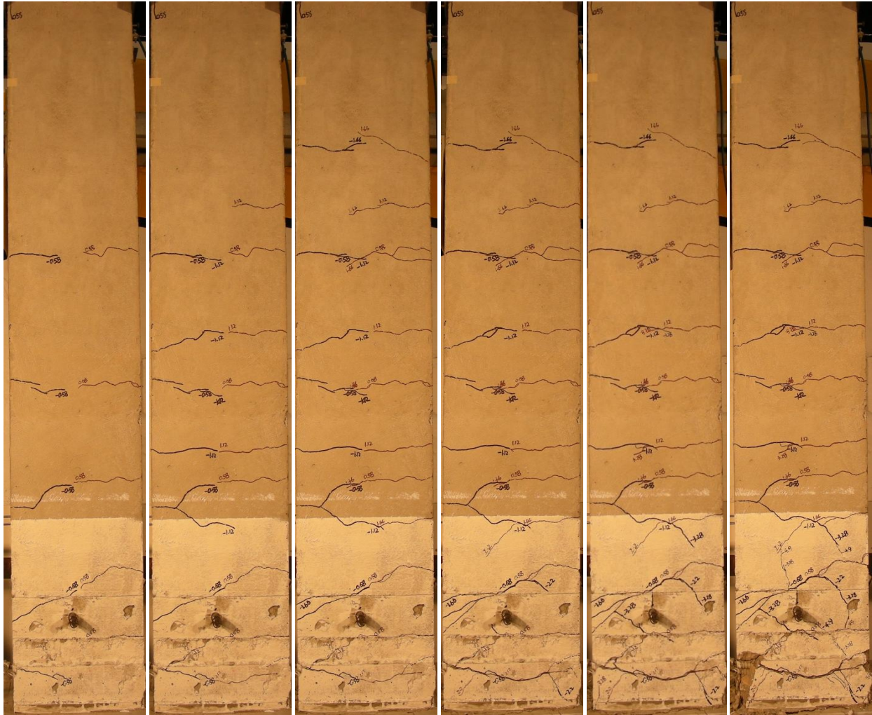
(a) \pm 0.58 in. (b) \pm 1.12 in. (c) \pm 1.66 in. (d) \pm 2.20 in. (e) \pm 3.28 in. (f) \pm 4.8 in. Figure A.21-Crack map under various loading cycles (S1)
