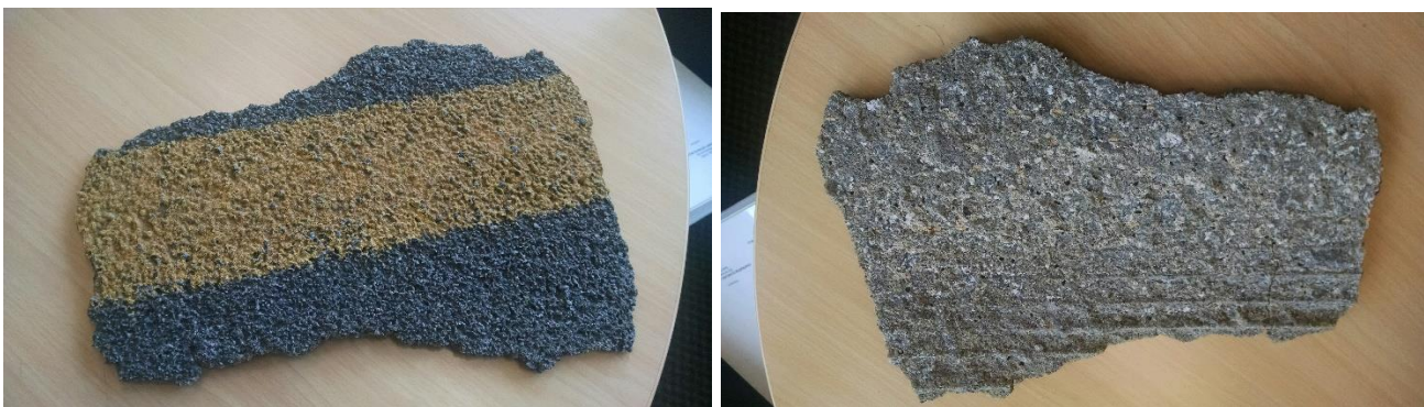
Figure 53. Delaminated multi-lift polyester overlay (from the Marquette Interchange ramp).
