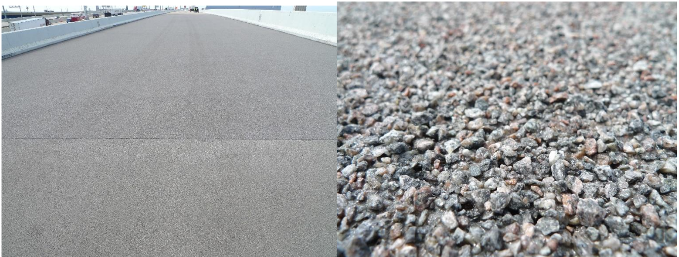
Figure 31. Marquette Interchange ramp after placement of four different thin polymer overlay systems (A through D).
