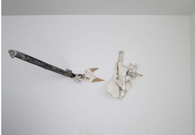
Figure 5.6. Above ground storm shelter in Moore that was perforated by flying debris.
